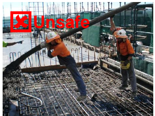
Figure 4 – Workers stretching hose for additional reach. This is an unsafe work practice.
